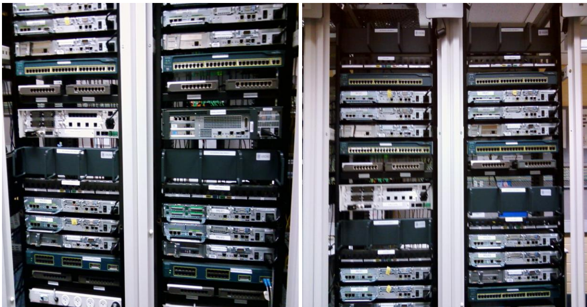
Figure 2: Equipment racks in the computer networking laboratory at ECU
