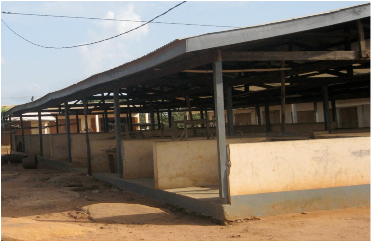
Photo 6.1: The deteriorating Tease CBRDP Market
