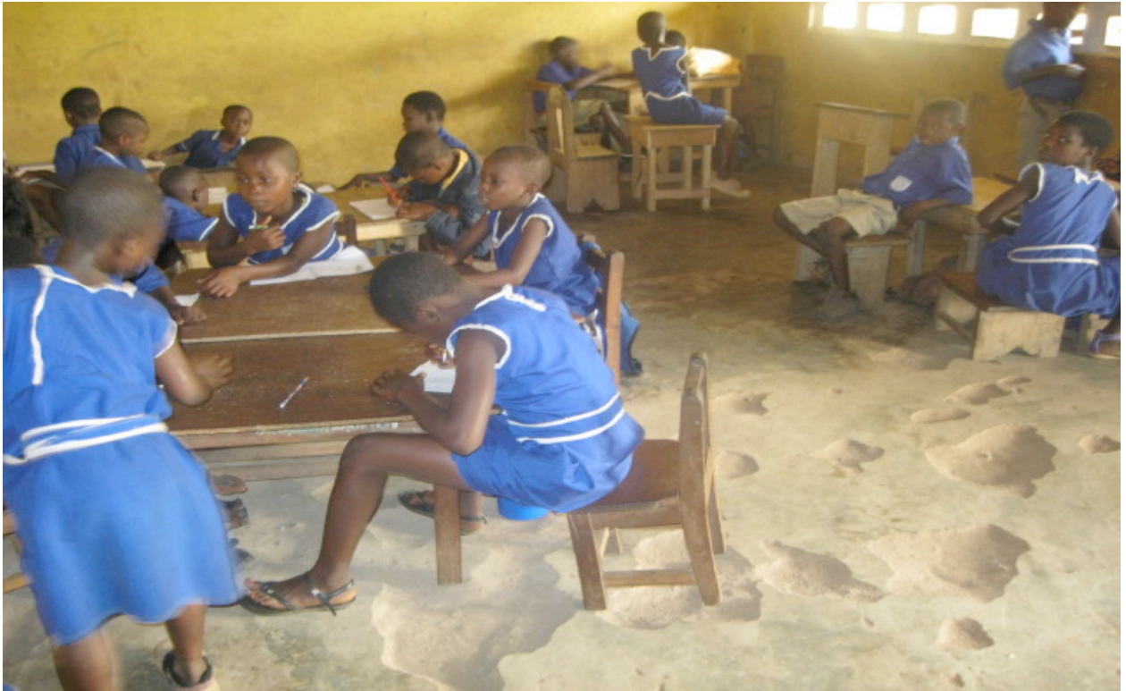
Photo 6.4: The deteriorating state of the Tashie Presby School.
